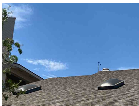
Unprotected glazed openings skylights
