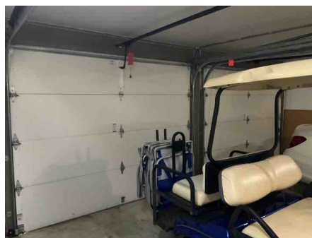
Unprotected garage doors
